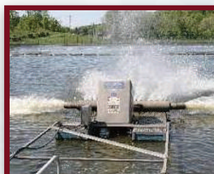
Typical UEE Compatible Aeration system through Surface Aerators
